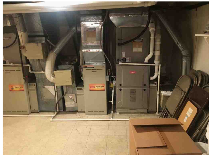
BASEMENT MECHANICAL ROOM
