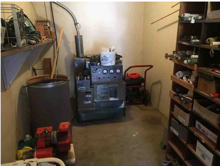
STORAGE AND GENERATOR ROOM BELOW THE GARAGE
