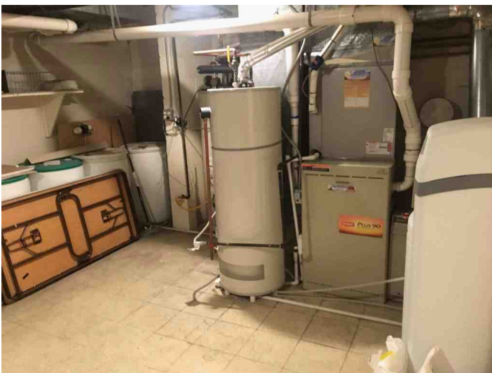
BASEMENT MECHANICAL ROOM
