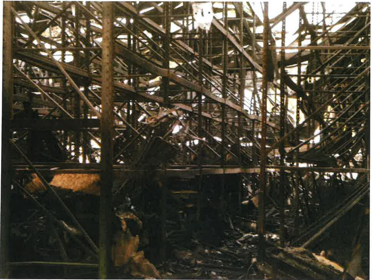
Photo 9. Storage racks in warehouse post fire. Storage racks were filled with various furniture and mattress items. Note the extent to which the storage racks filled the warehouse which gives an indication of the volume of merchandise and the fuel load inside the 15,600 square foot warehouse. The warehouse measured approximately 130 ft. by 120 ft. and was 29 ft from floor to roof. (Photo – NIOSH.)
