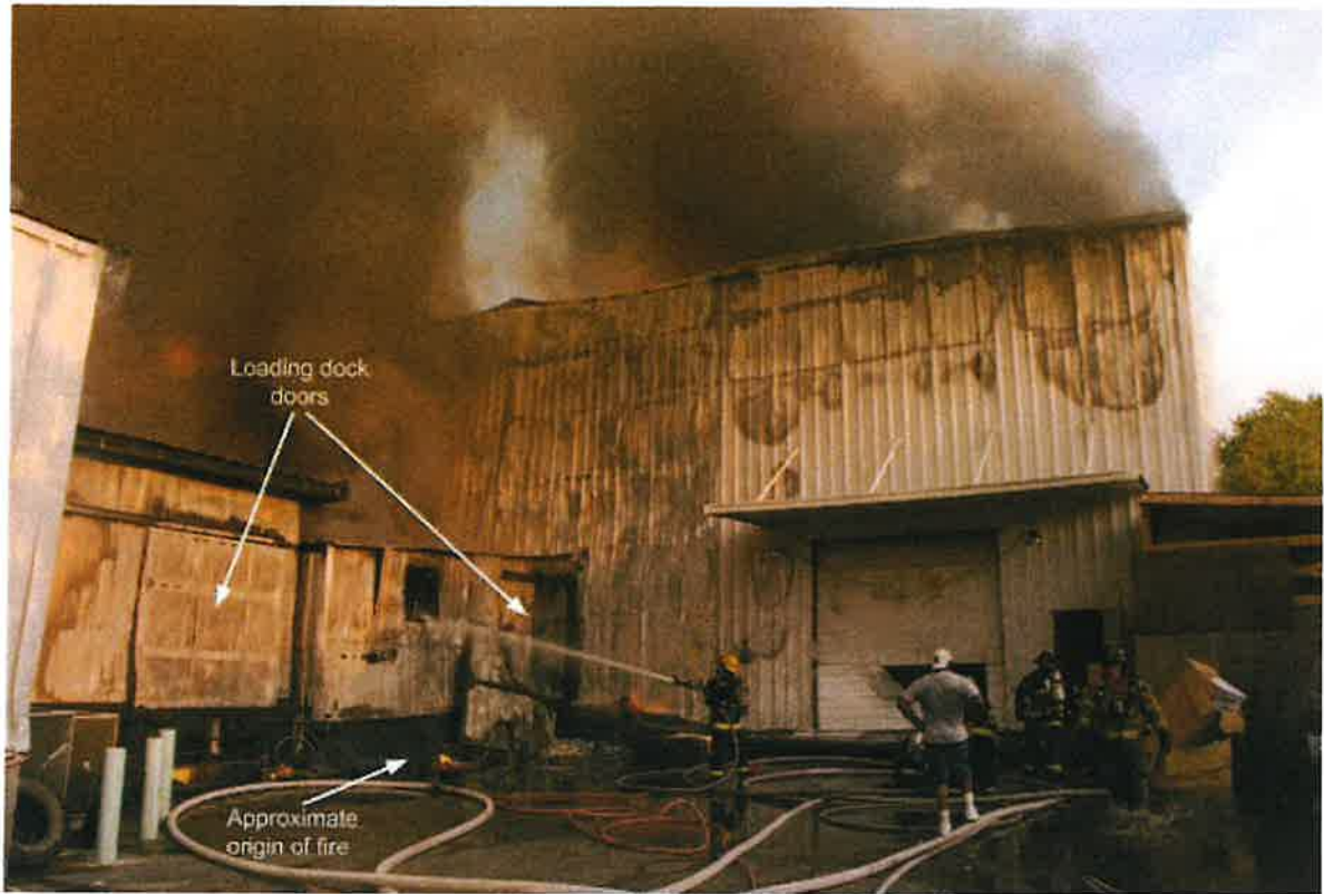
Photo A-2. Time is approximately 1936 hours. Loading dock area approximately 20 minutes after first crews arrived on scene. There is heat damage to metal siding on loading dock and warehouse. There are two Loading dock doors. There is an approximate origin of fire in the corner. (Photo courtesy of Police Department, Bill Murton, photographer.)
